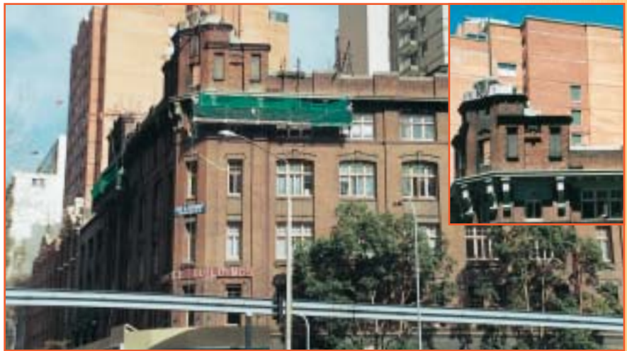
The Commerce Building during the repair stage. (Inset) The recently repaired sections.
