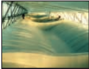
Sikafloor®-400N Elastic on commercial building
