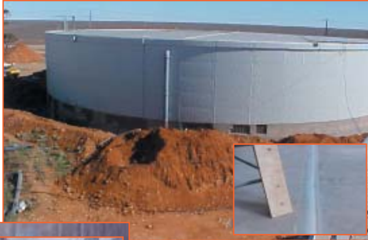
Water tank to be repaired (Inset: Sikadur-Combiflex)
