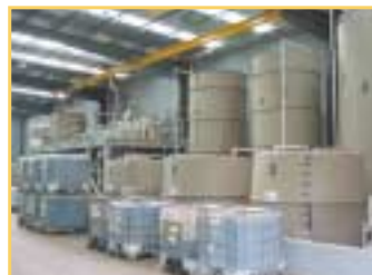
Admixture tanks at Keysborough, Melbourne
